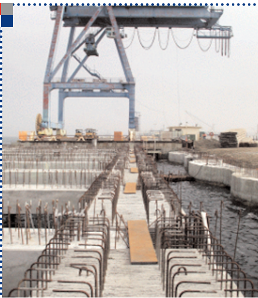
Crane Rail Beams System
